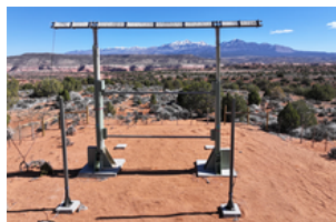
WETA Installation in Moab, UT
